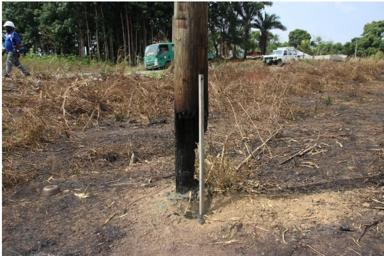
A pole damaged by bushfire
