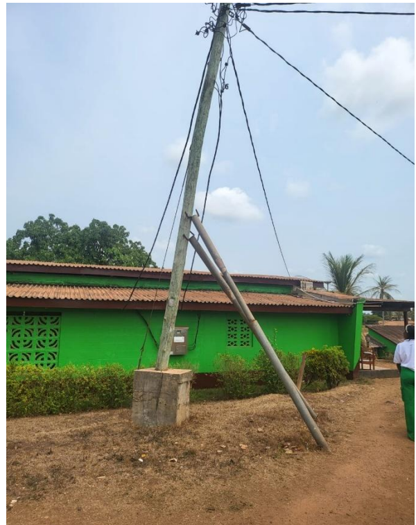
A broken LV pole
